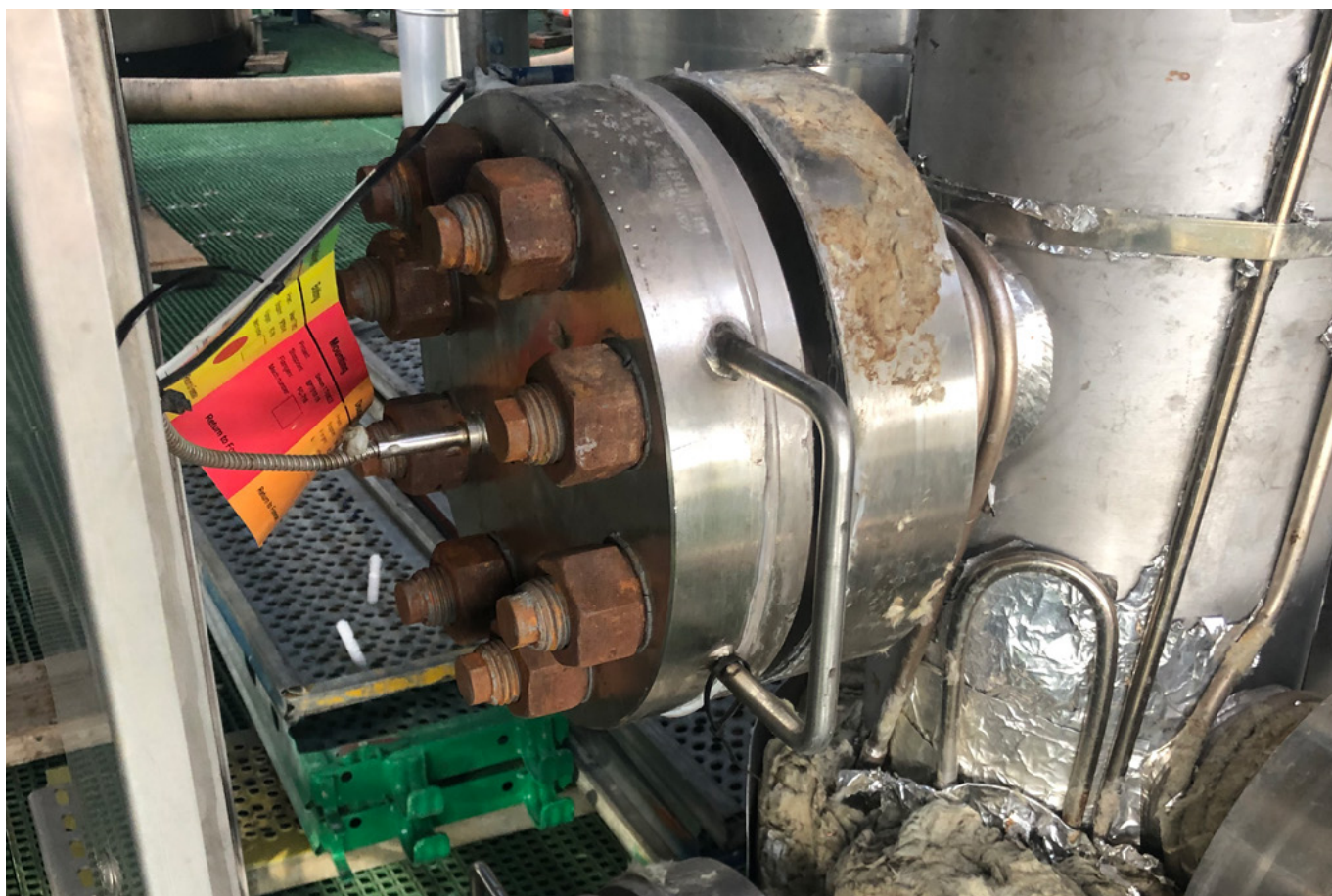
Diaphragm seal systems that were reintroduced into the process included relevant design improvements, such as added lifting handles for easier and more controlled placement of the very heavy 3” cl 2500 flanged EXT type seals.
